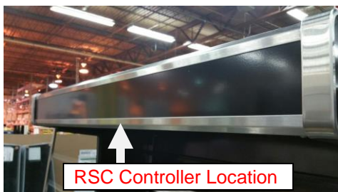
Figure# 1 : Location of the controller
